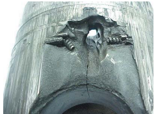
Fig. 2.7.11 Destruction of the crown and the pin boss region, due to irregular function of injection nozzle
